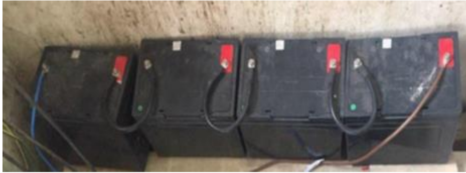
Figure 3: Battery bank of four batteries in series
