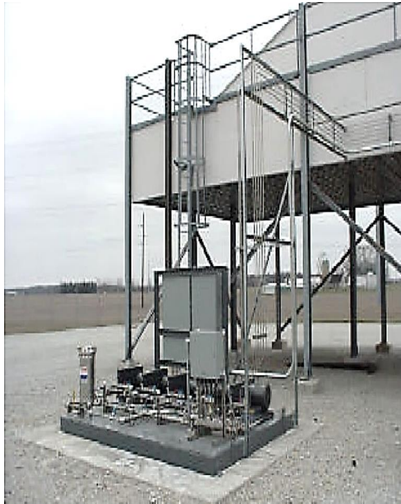
Figure 1. Typical fogging skid with high pressure. Here are the feed lines from the high-pressure pumps to the intake system [39]
